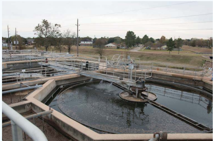
Figure 3-4. Photograph of Greatwood WWTP
